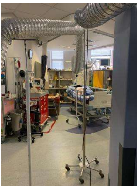
Figure 1: Duct pipes held up by IV stands.
